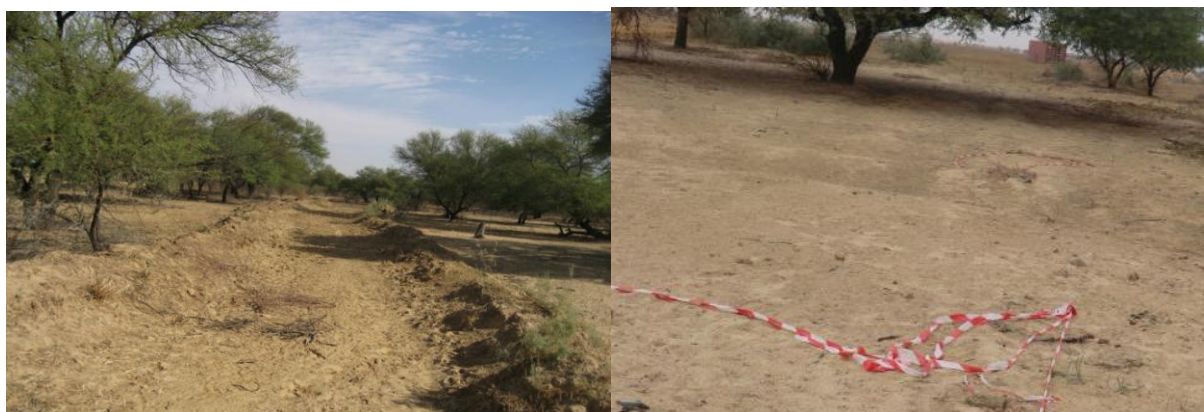
In 2010, the AIV removed obstacles in the bed of the Yéti Yone marigot to allow water to flow to the Grande Mare (left picture, Mbelele Mbaye in 2011, looking to the North - East). In Feb. 2015 a new bridge is being installed near Mbelele Mbaye (view to the west) The Yéti Yone is temporarily dammed here during these works (right picture).
