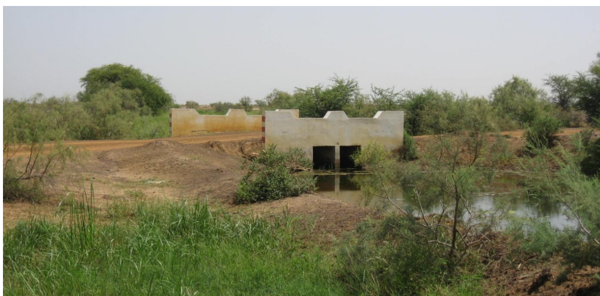
Pont Alain Daniel in Oct. 2012, was constructed with the help the local outfitter Alain Daniel to support the AIV and to allow for water in the Ndiael.
