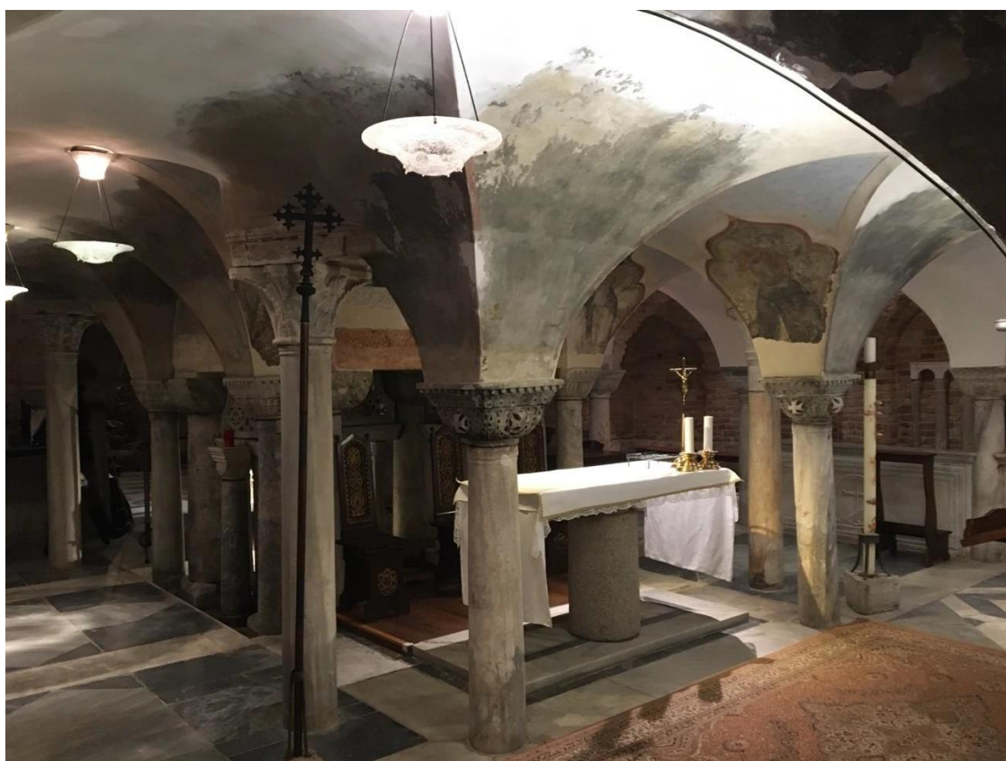
Basilica di San Marco. The crypta flooded – and after drying, the input of salt can be recognised on almost all surfaces. (City of Venice, Bernhard Furrer)
